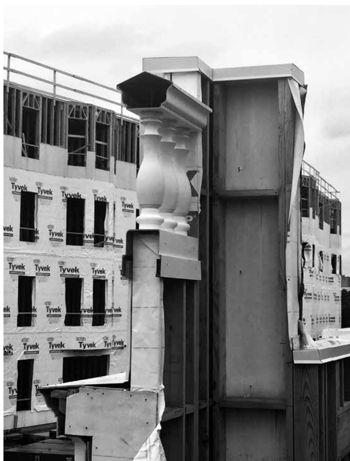
10 Extruded aluminium classical elements on a full-size wall mock-up at a housing construction site in Alexandria, Virginia (2017).
