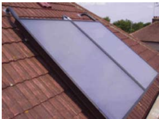
Figure 9. Passive solar hot water system on a residential roof top.
