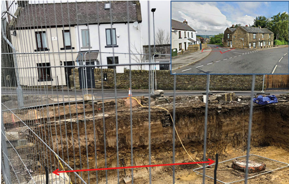
FIG. 13. Hoylandswaine. The excavated cellars of the Old Post Office. The red arrow marks the approximate 7 to 8 m width of the surviving Roman road visible in the side of the excavation. Inset: The Old Post Office before demolition, showing the road was well below modern ground level. The hollow red arrow denotes the route of the Roman road. (© D. Ratledge)
