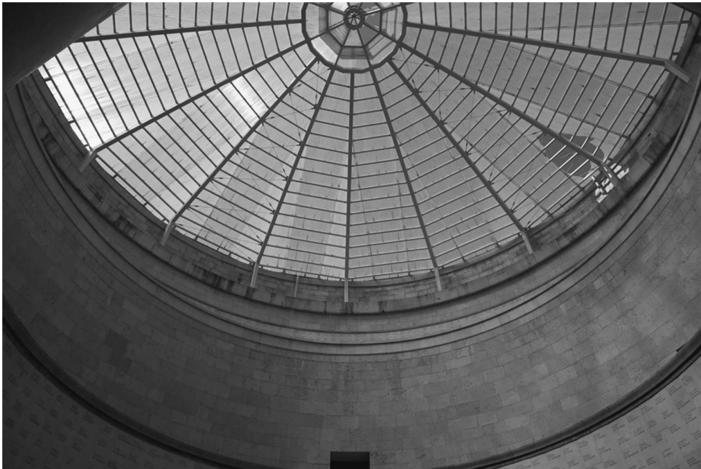
Figure 5. Signs of neglect at the ossuary of Oslavia, completed in 1935 (author’s photograph 2015).
