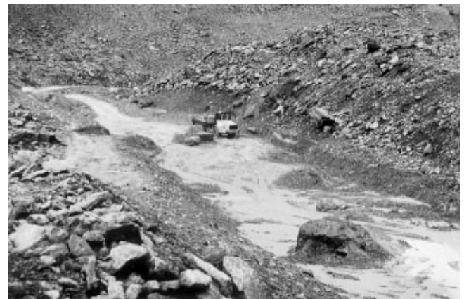
Fig. 13. Excavation of a drainage channel for ice-marginal Lake No. 3 (photo A. Kääb, 1995).
