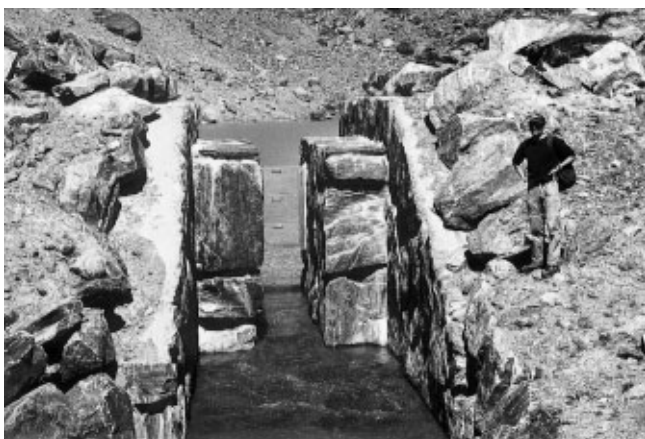
Fig. 14. New (lowered) flood-release (overflow) structure with regulating gates at proglacial Lake No. 1 (photo W. Haeberli, July 2000).
