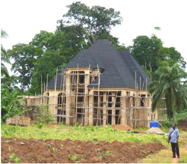
PLATE 2 Construction of a large residence adjacent to a sacred forest grove commonly used by monkeys. (Photograph: Lynne R. Baker)
