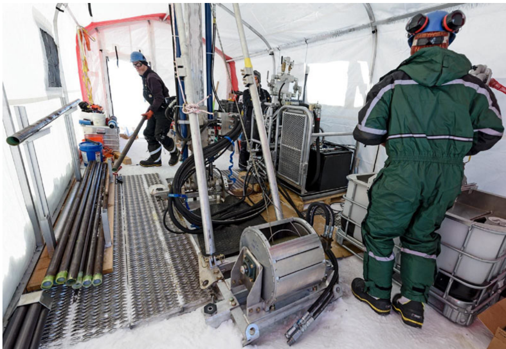
Fig. 16. Access hole drilling operations with the ASIG Drill system at Site 1 during the Pirrit Hills, Antarctica field project in 2016.
