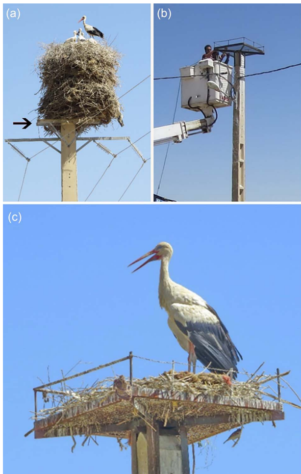
White stork Ciconia ciconia conservation project in central Iran: (a) reconfiguration of 20 kV medium-voltage power line (the arrow shows the original crossarm), (b) installation of first nest platform on 220 V low-voltage power pole, and (c) occupation of nest platform. Photos: Mahmood Kolnegari.
