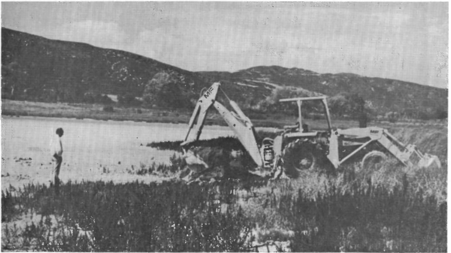
Trenching operations on margin of Elizabeth Lake, California. This sag pond virtually dried during the fall, 1977.
