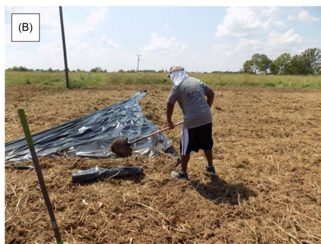
Figure 2. (A) Implementation of flooding treatments and (B) installation of 6-mil black tarp.
