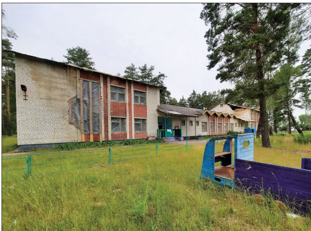
Figure 3 . Eastern facade of the Yahidne school, showing damage to the roof and walls caused by rocket strikes, 11 June 2023 (photograph by M. Lemiesz).
