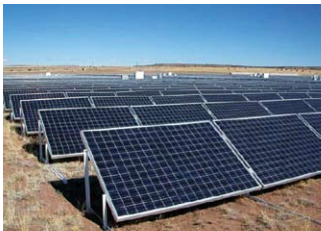
Figure 6. Two megawatt system installed at the Sacramento Municipal Utility District power station in Rancho Seco, Arizona.
